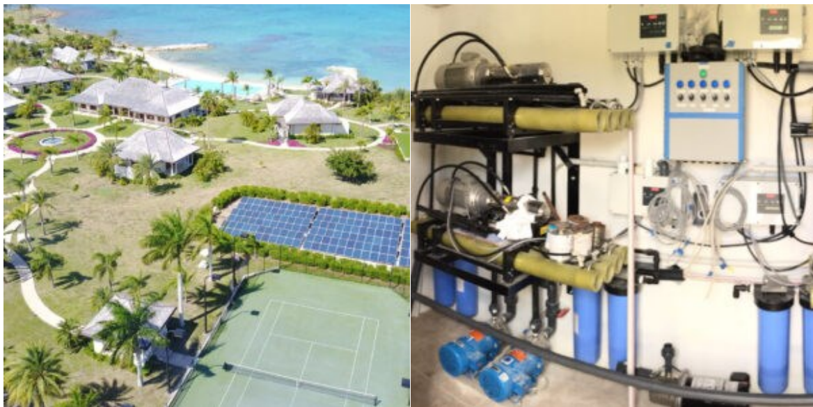
Figure 7 – Independent water supply for a large estate at Jumby Bay, a private island off the coast of Antigua (Source: https://aqsep.com/ )
