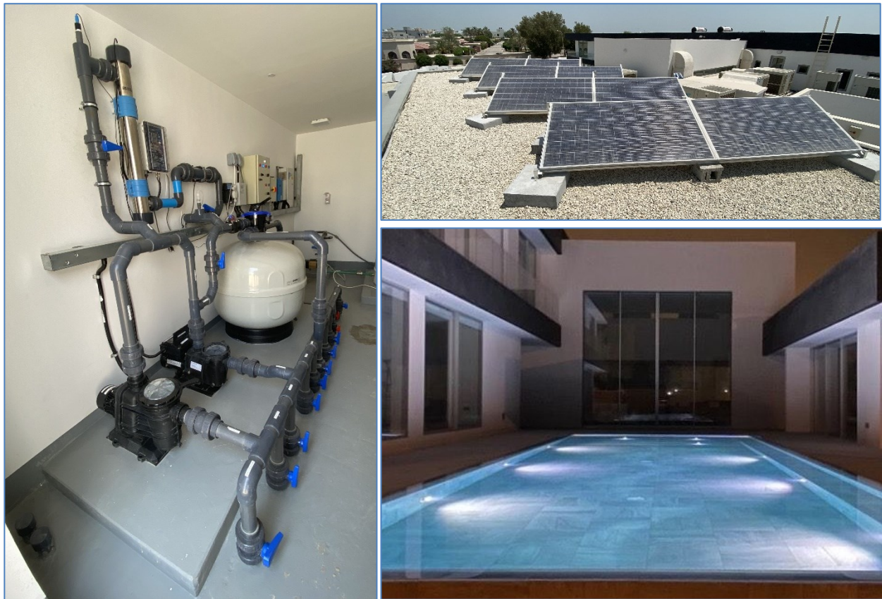
Figure 3 – The combo figure shows a pool pumping system installed in Bahrain (Source: Lorentz – https://www.lorentz.de/ )
